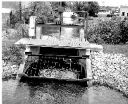
Smaller gate at Lakeshore Drive regulates flows through Feeder Canal that receives effluent from Canandaigua sewage treatment plant.
