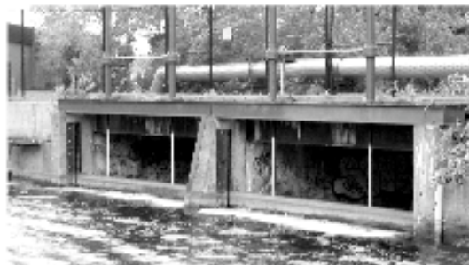
Larger gate on main channel regulates flows from Canandaigua Lake into Outlet.
